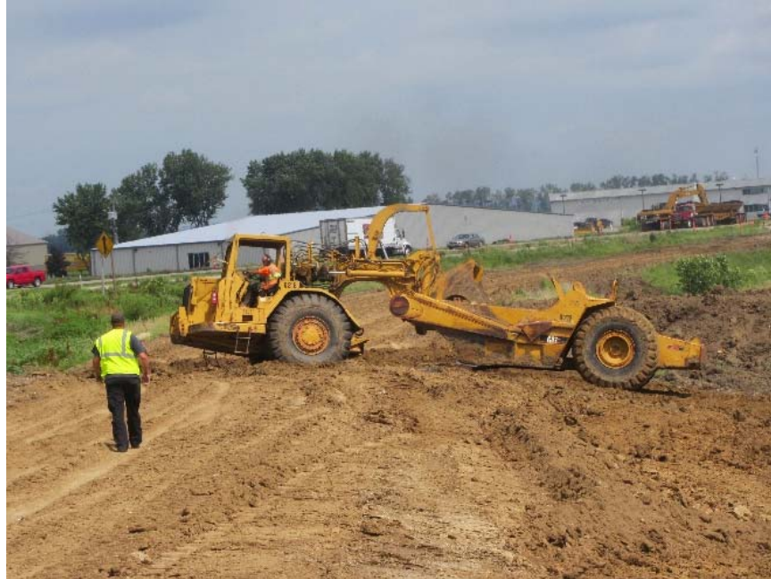
Figure 88. Mills County Project 5: Caterpillar 621E scraper used to collect and place loose fill materials
