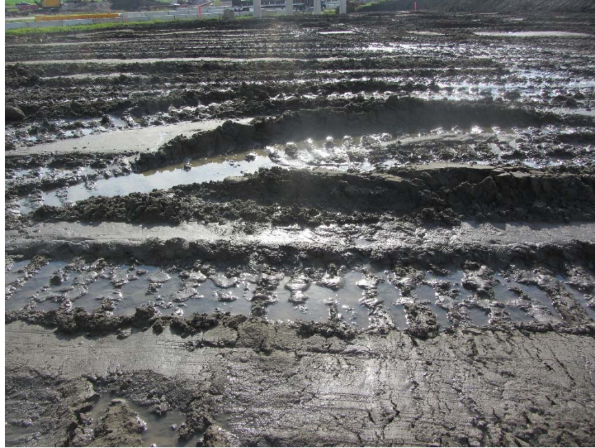
Figure 115. Woodbury County Project 7: Seepage at the construction site
