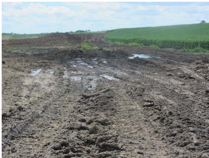
Figure 57. Linn County Project 3: Seepage at the construction site
