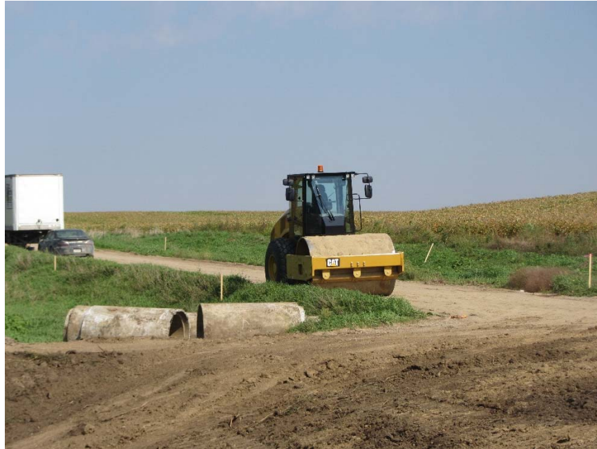
Figure 144. Woodbury County Project 9: Caterpillar CS56 series vibratory smooth drum roller used for soil compaction
