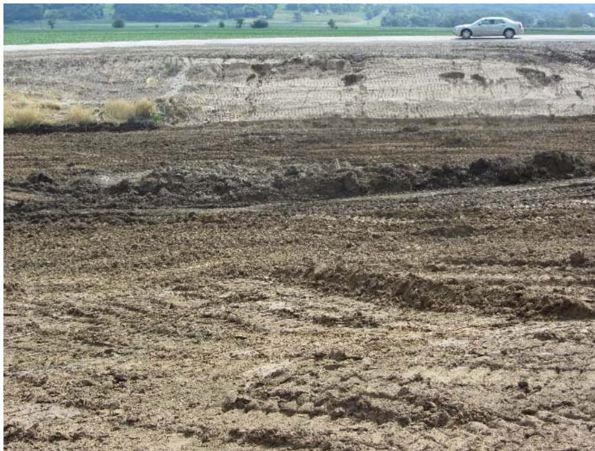
Figure 91. Mills County Project 5: Very wet materials in the center of the construction site
