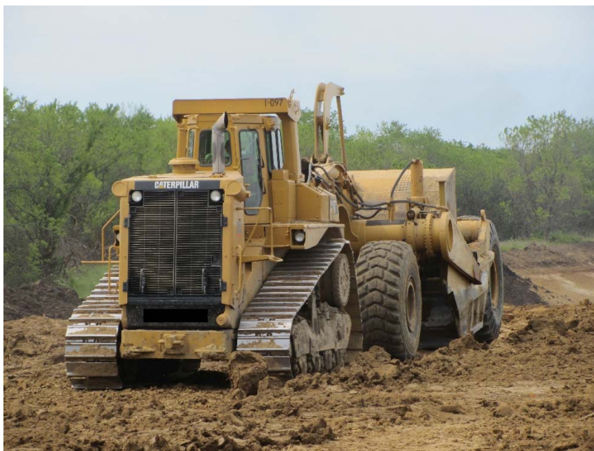
Figure 39. Warren County Project 2: Caterpillar MT-35 scraper used to collect and place loose fill materials
