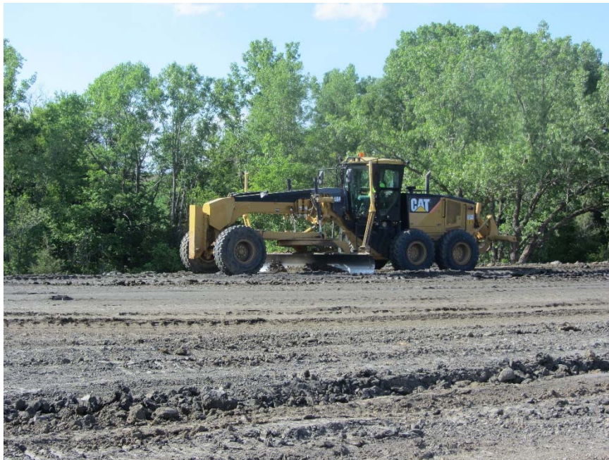
Figure 56. Linn County Project 3: Caterpillar 14M motor grader used to level the embankment surface
