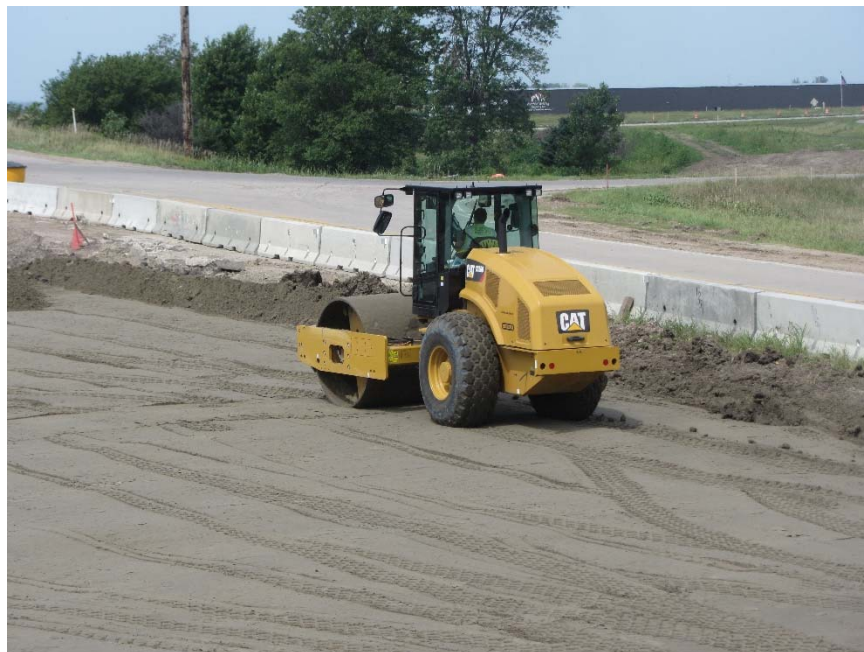
Figure 114. Woodbury County Project 7: Caterpillar CS56B vibratory smooth drum roller used for soil compaction
