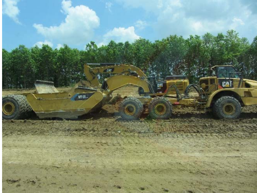
Figure 21. Polk County Project 1: Caterpillar MT-35 scraper used to collect and place loose fill materials
