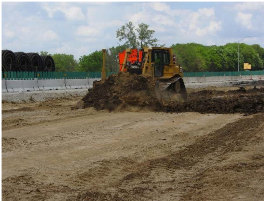
Figure 25. Polk County Project 1: Caterpillar D6T dozer used for grading and lift thickness adjustment
