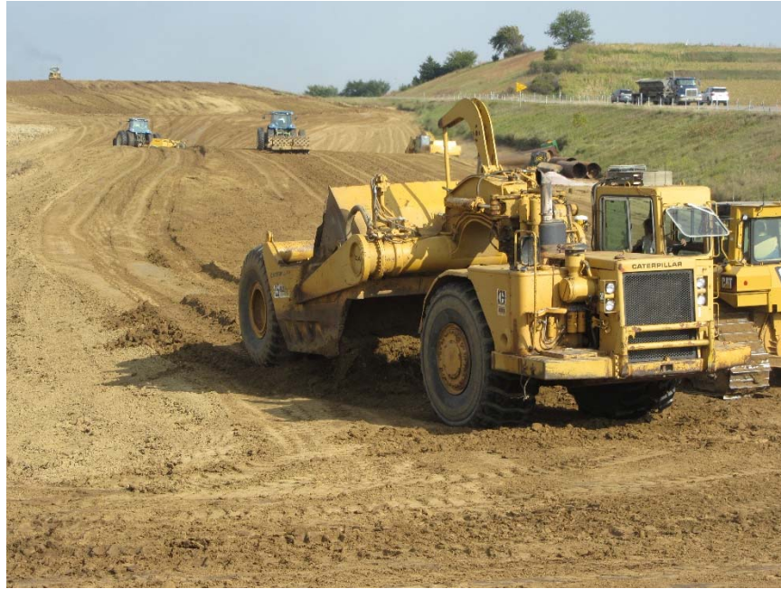
Figure 141. Woodbury County Project 9: Caterpillar 631D motor scraper used to collect and place loose fill materials
