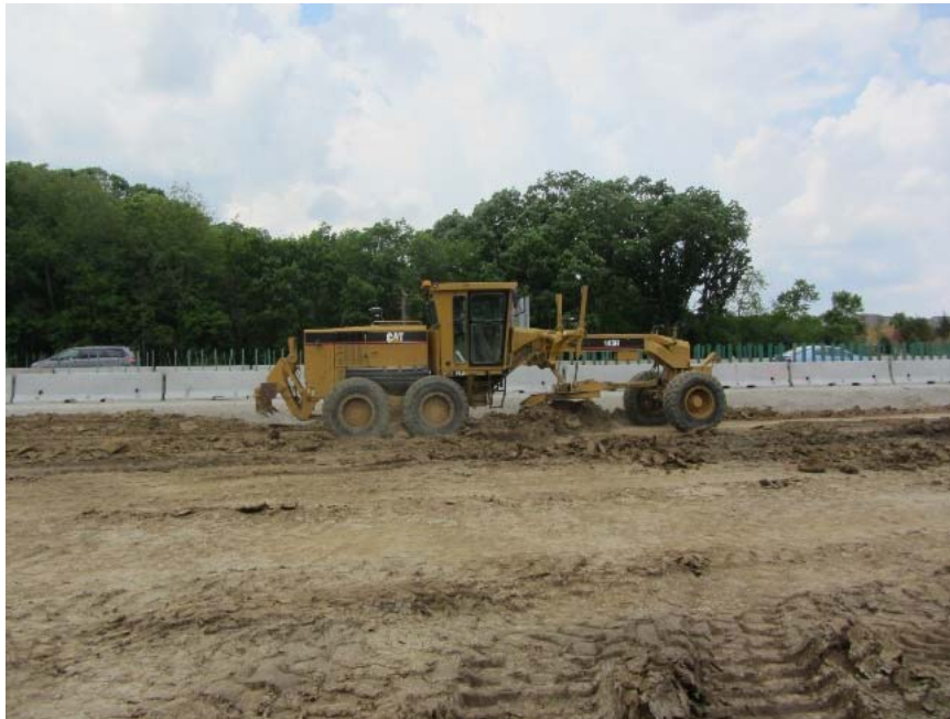
Figure 23. Polk County Project 1: Caterpillar 143H motor grader used to level the embankment surface
