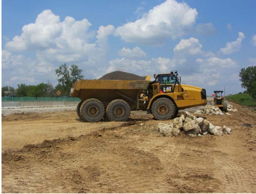
Figure 22. Polk County Project 1: Caterpillar 740B dump truck used to place loose fill materials
