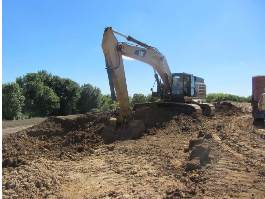
Figure 126. Scott County Project 8: Caterpillar 349E used to excavate materials from borrow source
